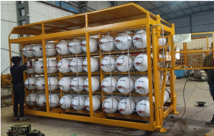
CNG cascade — manifold and valve assembly
